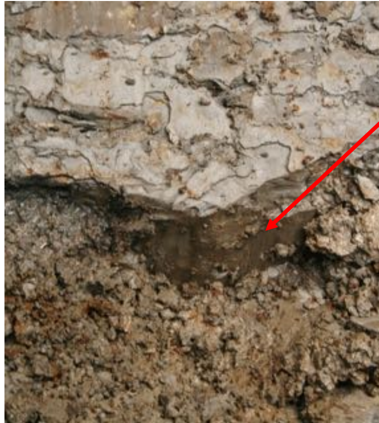
Displacement of Foundation Wall – Predominantly Lateral
