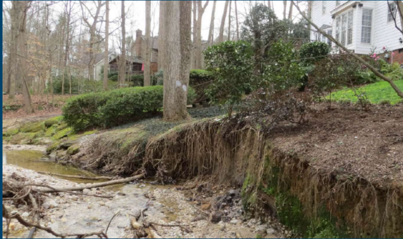
Major Erosion Drainage Assistance
